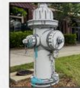
Fire Hydrants | Smyrna, GA
